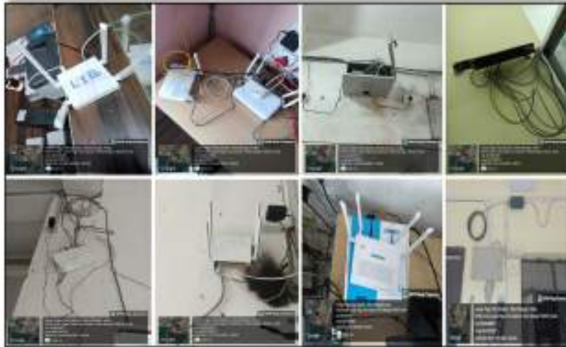
Installed Routers facilitating Wi-Fi enabled campus
